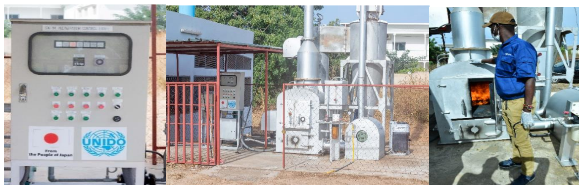
Source: CHUWA Incinerator for Medical Waste, Project records, 2021
