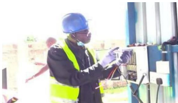
Country: Kenya Company: Kinsei Sangyo Co., Ltd. On-site assembly and installation work
